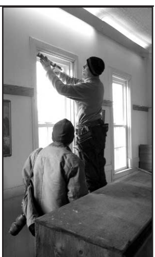
John Flaherty and Mike Buote of Capeway Aluminum install new windows at the Little Red Schoolhouse.
